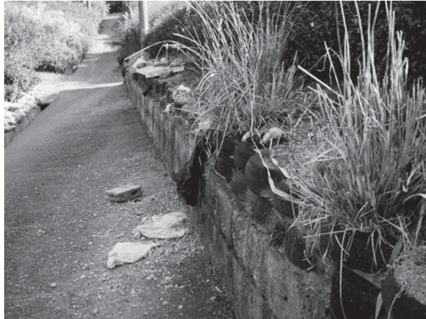
Picture1: Broken blocks in Makinohara City Photo:Takabayashi (2016)
